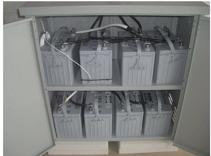
Figure 1. Residential Photovoltaic Battery Backup – critical for extended outages.
